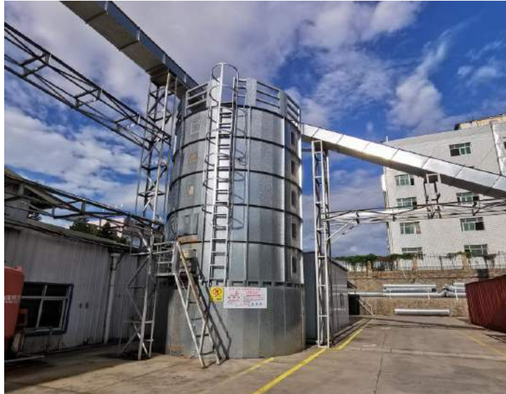
Wood processing Dusts treatment
