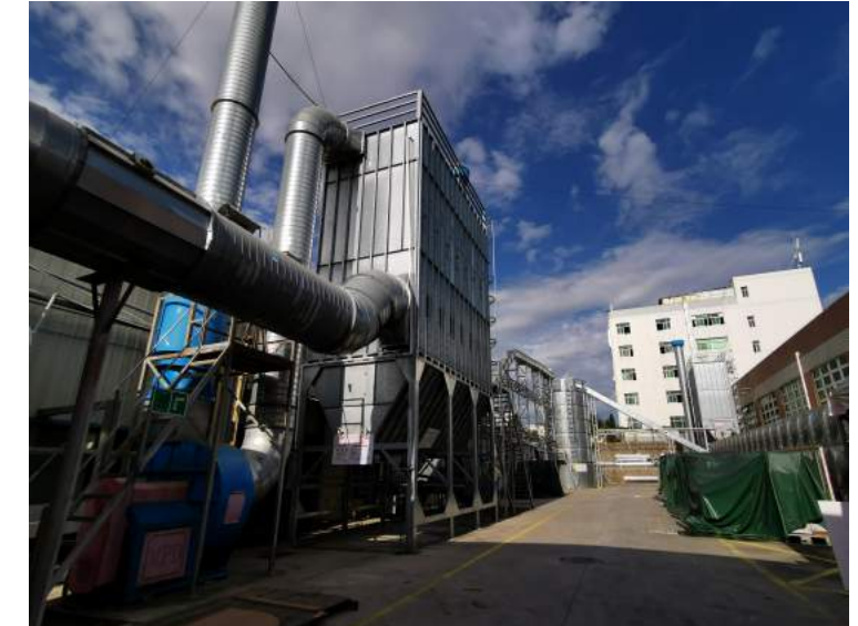
Wood processing Dusts treatment
